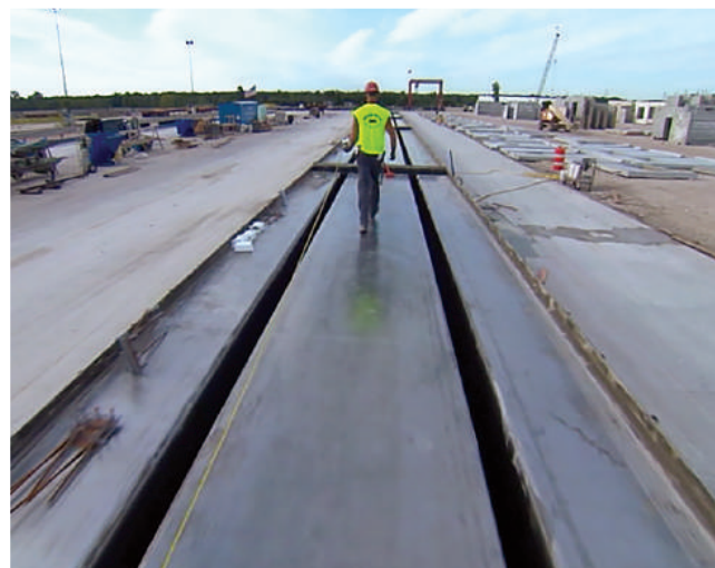
Figure 1.1.2. Long-line, prestressed, double-tee casting bed is one key to both economy and quality.
