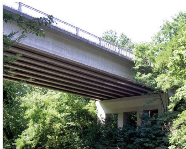
Figure 1.1.1(b). In 1990 the Walnut Lane Memorial Bridge was rebuilt using pretensioned, prestressed girders.
