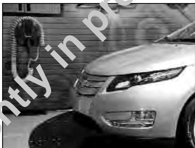
Figure 1.1.1 Electric vehicle supply equipment (Courtesy of NECA)
