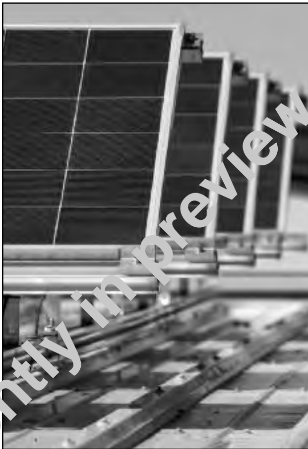
Figure 1.1 Typical roof-mounted array of a photovoltaic power system (Photo: iStock)
