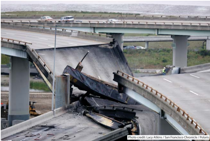
Figure 2-9. MacArthur Maze after failure.
