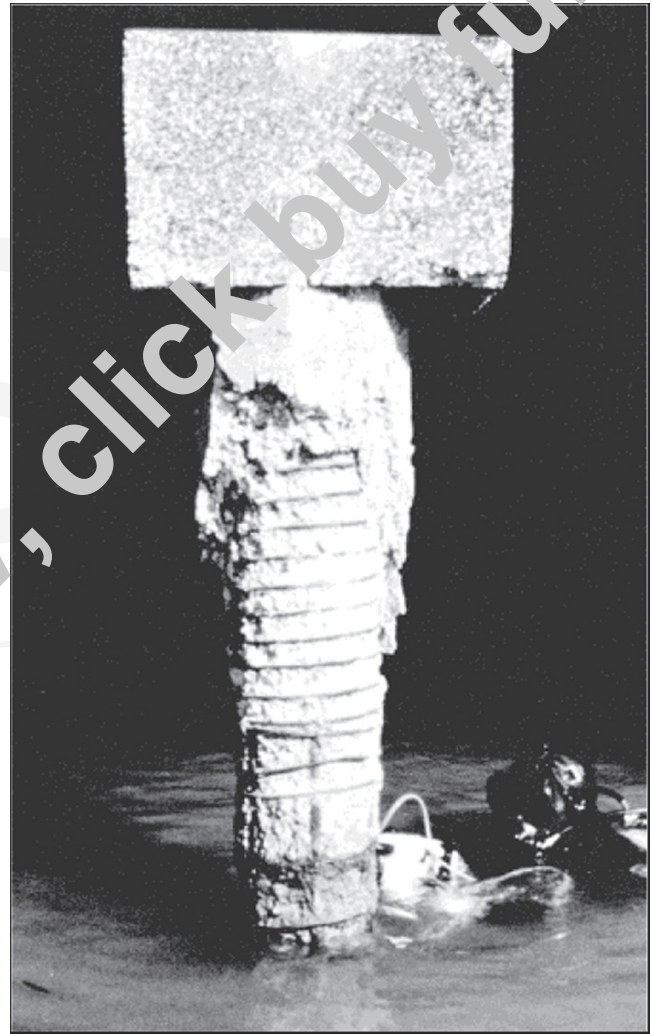
Fig. 1.1b—Deteriorated pile in tidal and exposed zones (image courtesy of M. J. Garlich).
